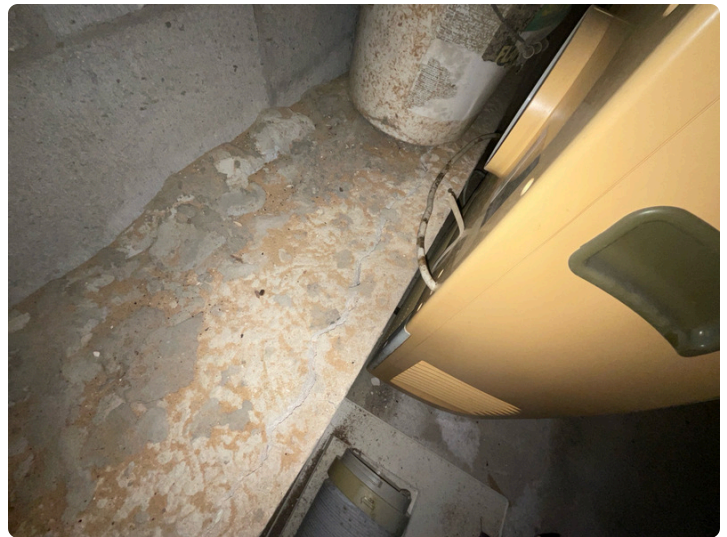
Crack/spall running along of wall
