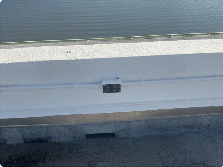
Exposed electrical outlet on parapet wall
