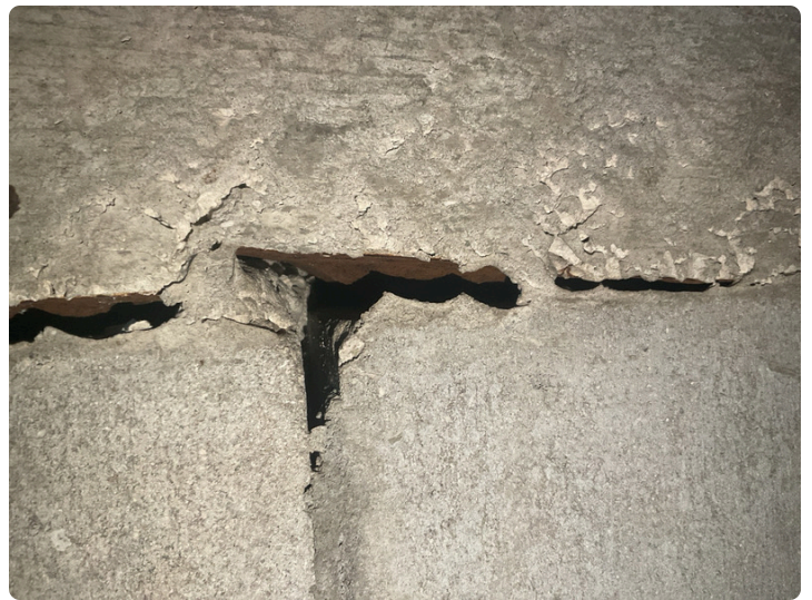
Spalling concrete/exposed metal in basement wall
