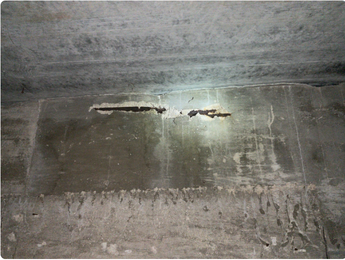
Spalling/exposed metal in basement
