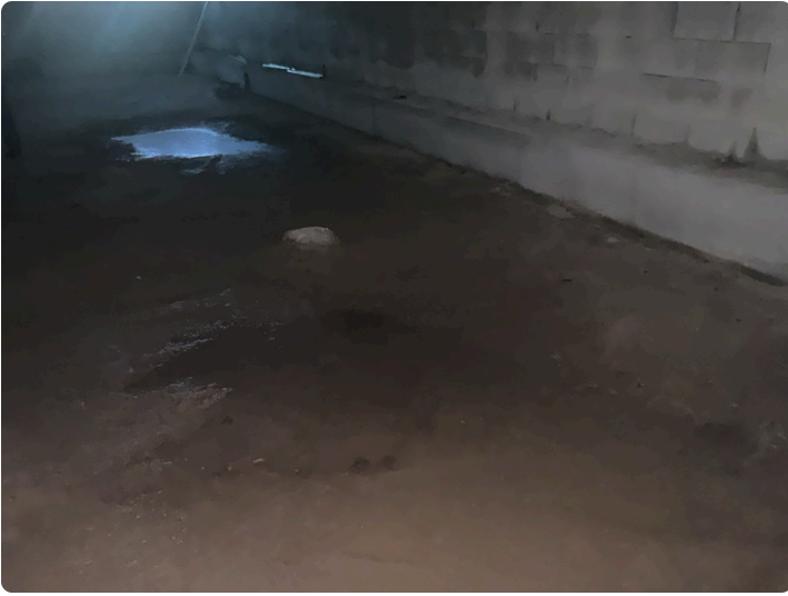
Sediment buildup in basement
