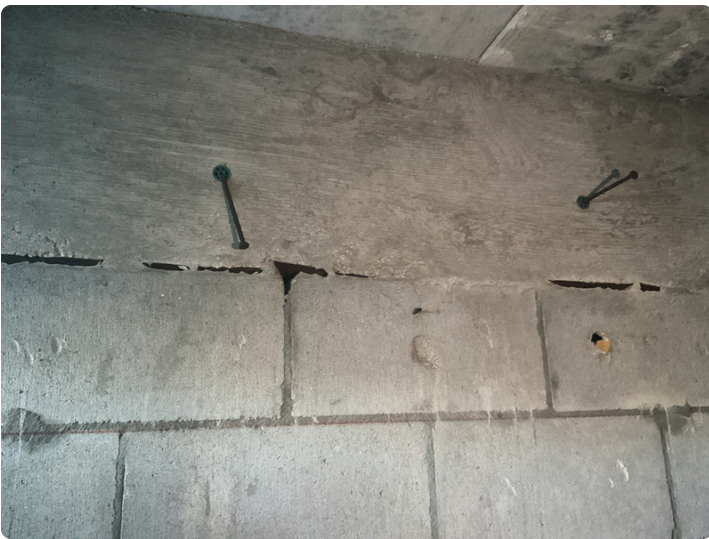
Spalling concrete/exposed metal
