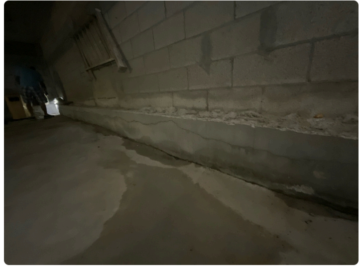
Spalling/crack running along length of room
