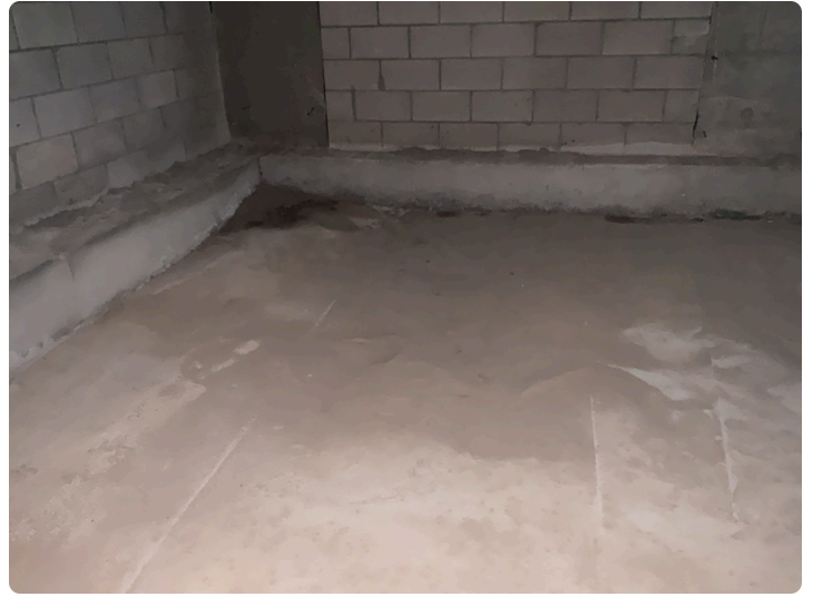
Sediment building in basement sediment buildup in basement
