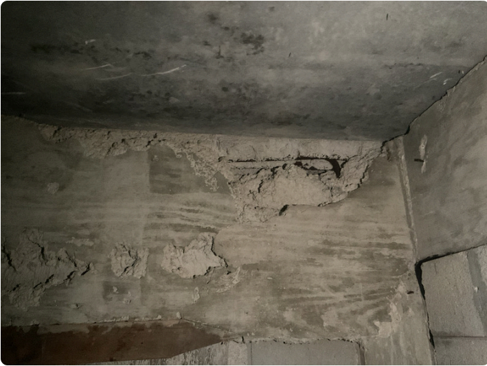
Potential spalling concrete
